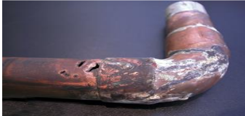
Gambar 5.3 korosi Erosi ( Erosion Corrosion )
